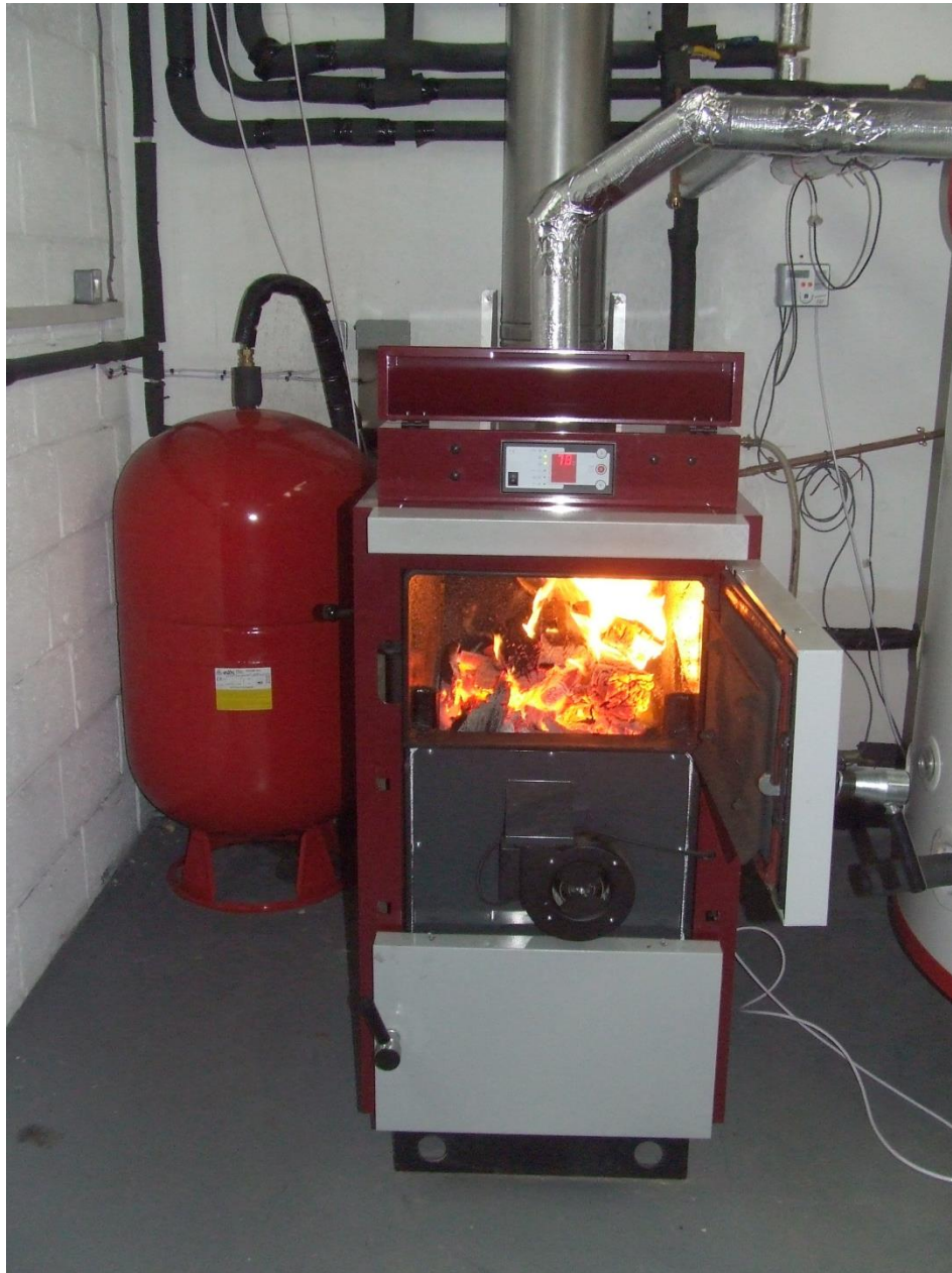
Biomass boiler with the top door open
