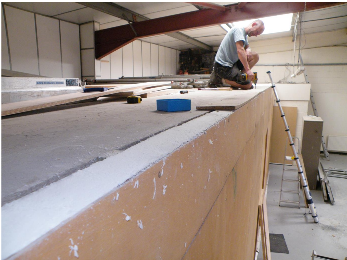
Insulation on the office wall, covered with fire proof plywood.
