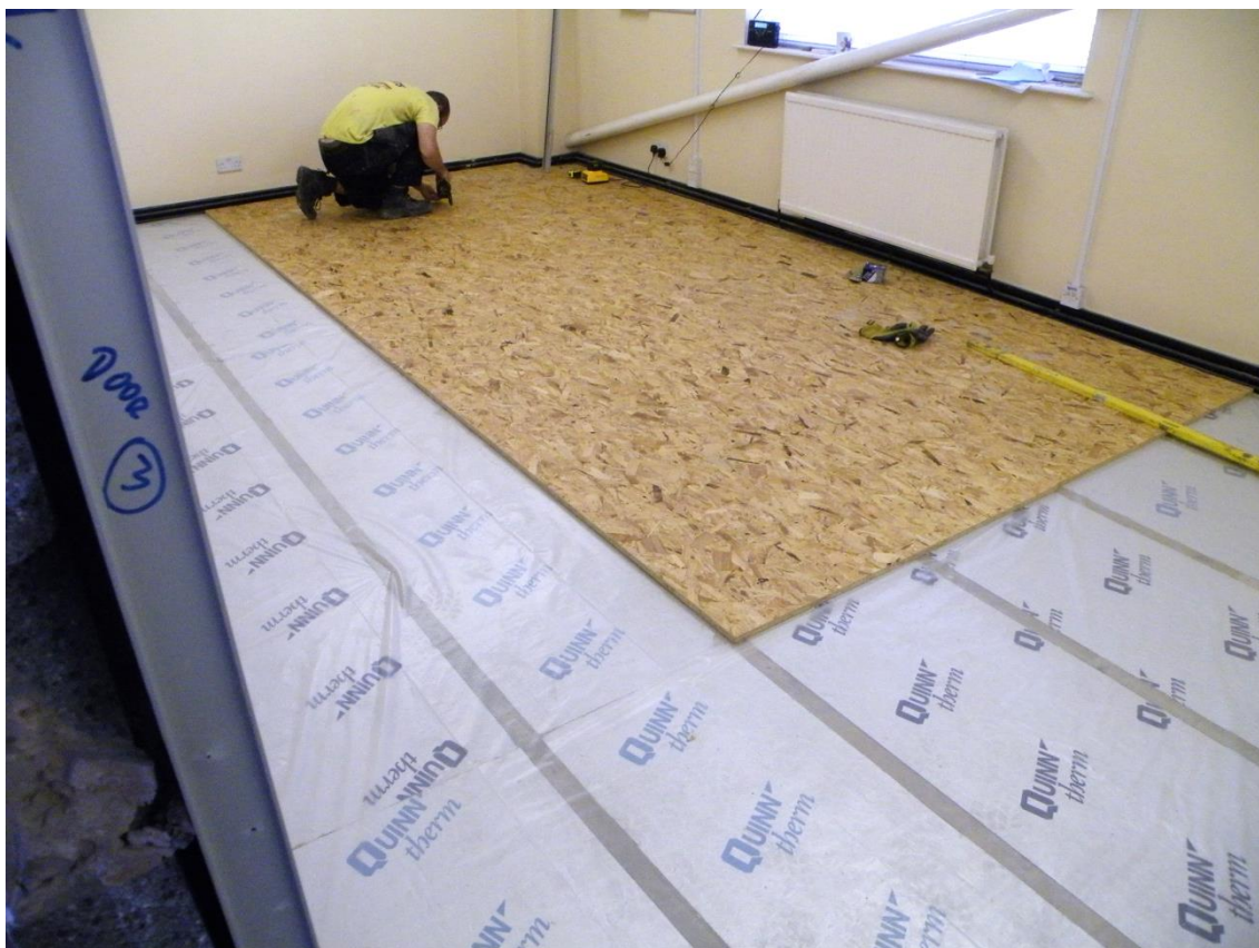
Insulation of the floor – polyurethane foam insulation covered with Orientated Strand Board.
